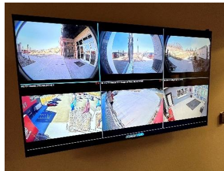
Fire Station camera monitor
