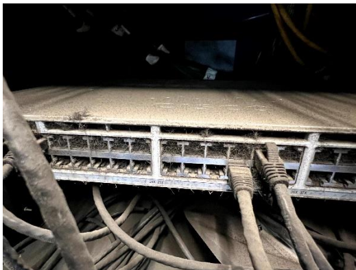
Dusty switch at Maintenance
