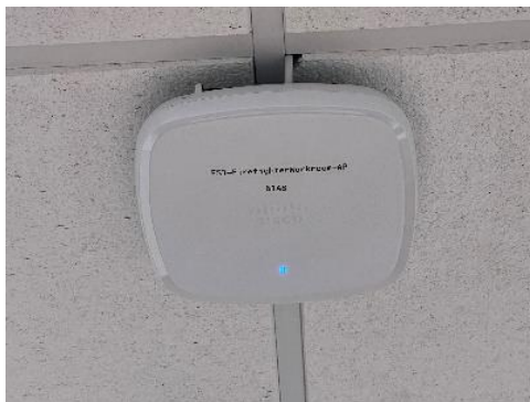
Access Point at Fire Station 1
