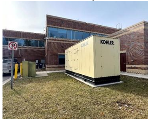
Power generator outside of the building
