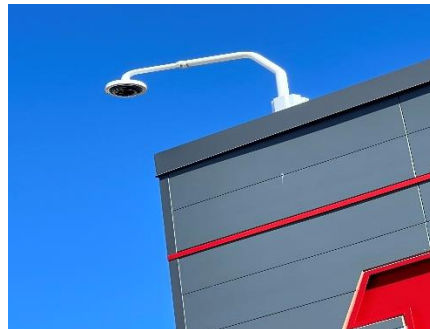
Exterior camera at fire station
