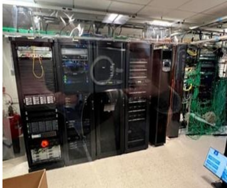
Front view of data center racks
