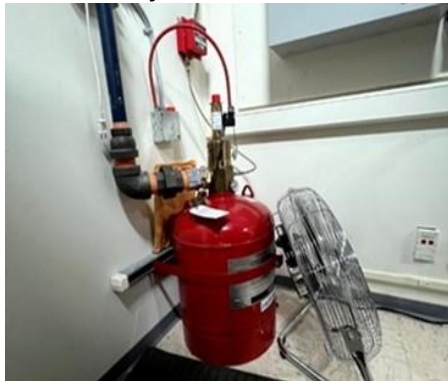
Fire suppression system
