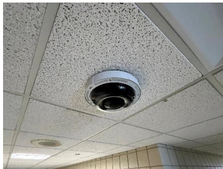
Interior camera at Maintenance Center
