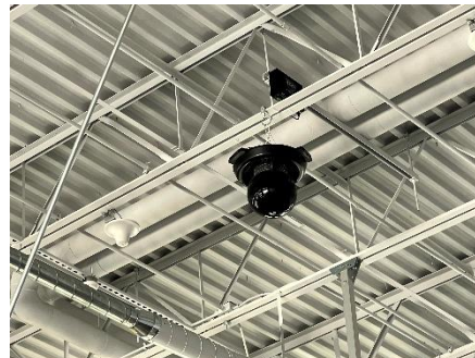
Interior camera at Ames Center
