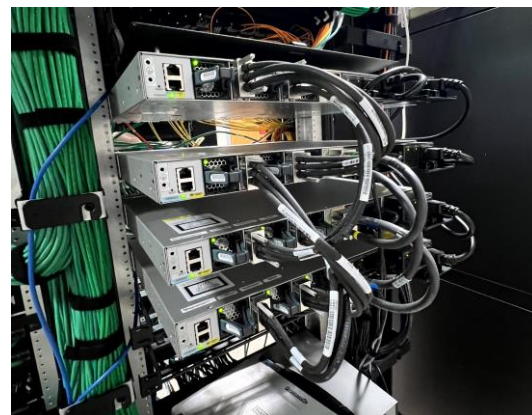
Switch stacking at City Hall
