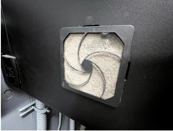
Clogged exhaust fan at Fire Station 1
