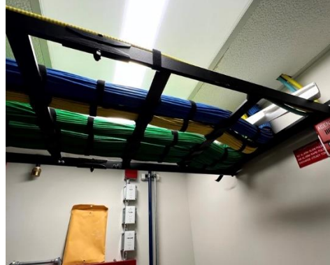
Ladder rack cable management
