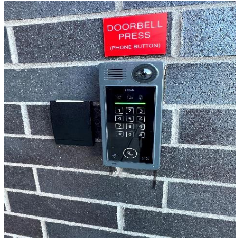
Video intercom at Fire Station
