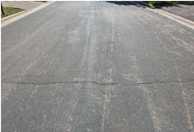
65 PCI (1 st Avenue, north of 130 th Street)
