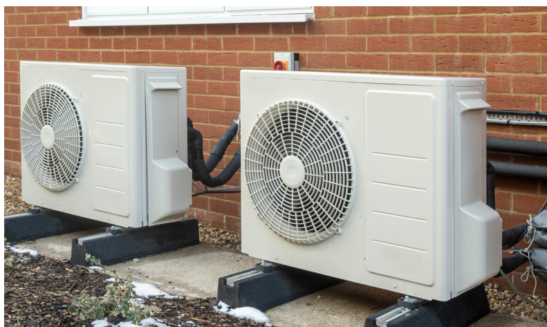
Air source heat pump units Photo courtesy of Partners in Energy
