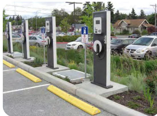
Electric vehicle charging station
